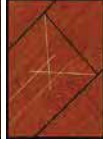
Picture 2: Change of damaged board is done in following way: First cut off the board with circular saw, but be sure that you set the sawing depth max. as thickness of wood flooring (in this case 14 mm). After that saw a "V" from each corner, and then saw from short end to short end to connect these "V" cuts.
