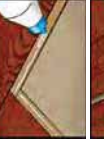
Picture 8: After that spread the glue on a free profile of neighbouring boards and on tongue on board.
