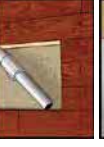
Picture 5: Vacuum carefully all wood dust and smaller wooden parts, to make area free and prepared for laying new board.
