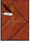
Picture 3: Remove the center section from the board. To be sure not to damage the neighbouring boards, use a chisel and manually extend the cut all to edges of neighbouring boards.
