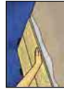
Picture 8: Go back along the row of boards, pressing them down against the subfloor (into the adhesive). Continue as in points 6-8.
