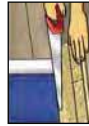
Picture 11: Doorframes can be removed and moved up, but it is usually easier to saw them off. Use a loose board as a height template and saw the frame with a fine-toothed saw. Push the floor under the frame (see also point 10) to shave off the part of the tongue which raises like a bump along the top of the outside edge.
