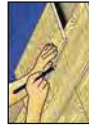
Picture 9: The final row of boards usually needs to be cut along its length. With its tongue against the wall, place the final board exactly on top of the frame with a fine-toothed saw. Push the floor under the frame (see also point 10) to shave off the part of the tongue which sticks out. Must still be cut off (to give the floor room to move). Saw and press down the final row of boards.
